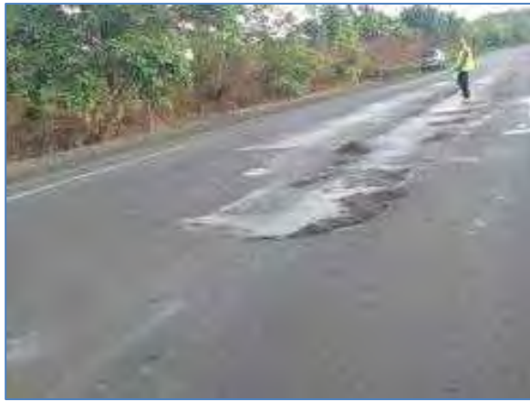
Bleeding & Patching at Km 127.700 RHS
