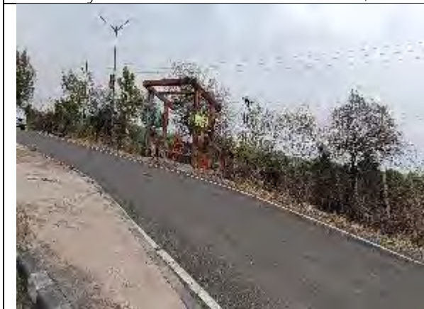
Damaged bus Shelter at km 127.585 LHS
