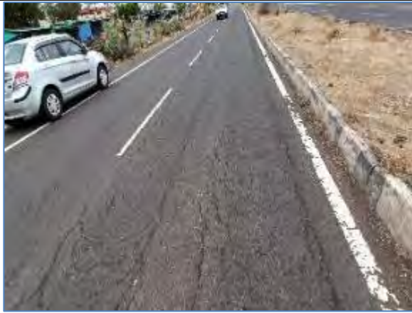
Rutting at Km 113.600 RHS
