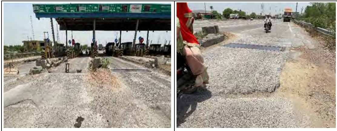
Figure 2.3: Rigid Pavement Condition
