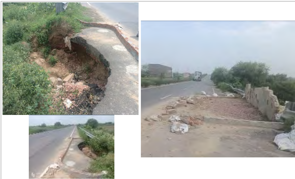
Photo 4: Road subsidence along the National Highway
