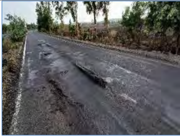
Shoving at km 125.600
