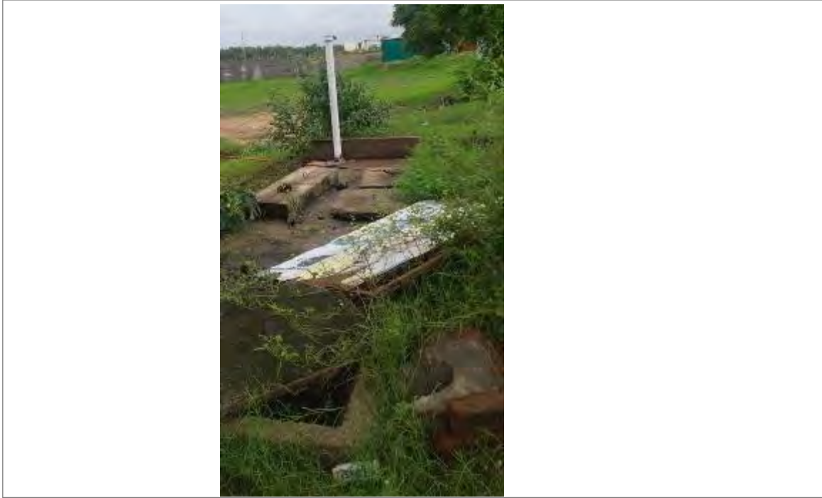
Photo 11: Septic tank in the toll plaza premise
