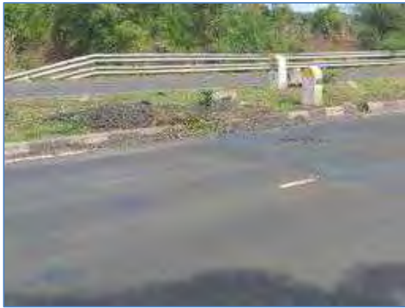
Pothole at Km 143.300 LHS
