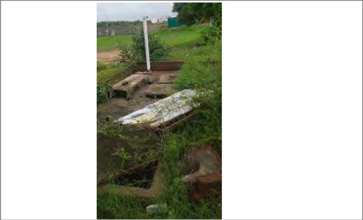
Photo 11: Septic tank in the toll plaza premise
