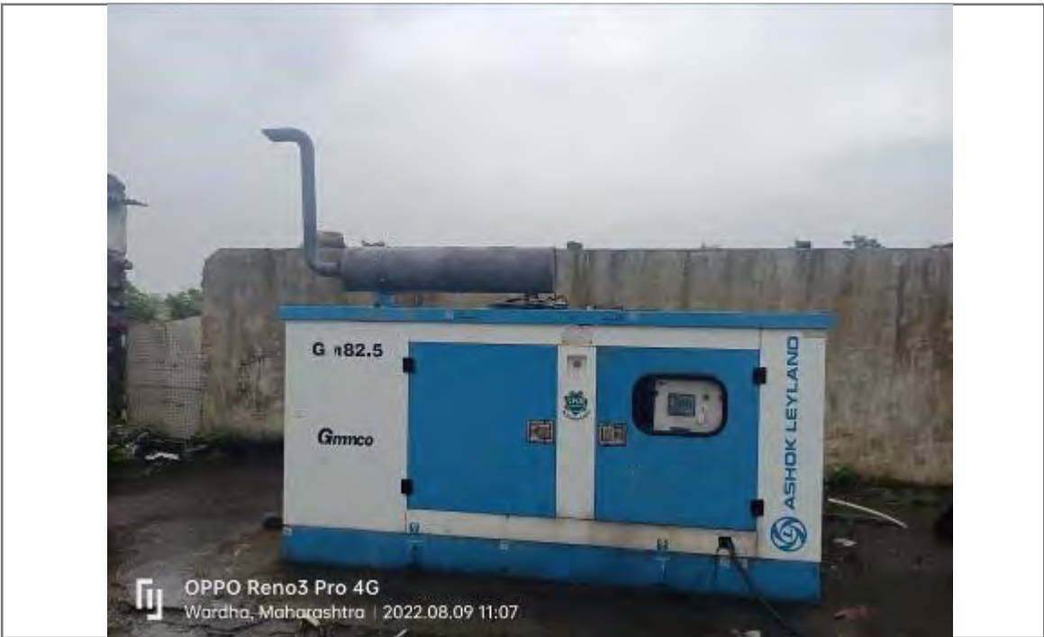
Photo 11: Diesel Generator at the toll plaza
