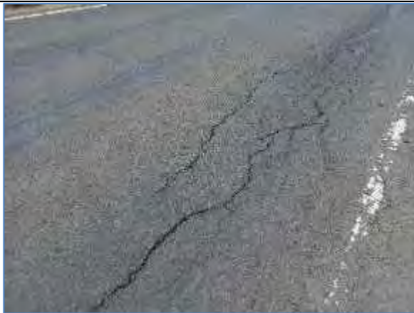
Longitudinal cracking at Km 59.100 RHS
