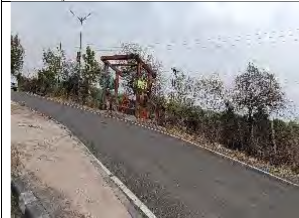
Damaged bus Shelter at km 127.585 LHS
