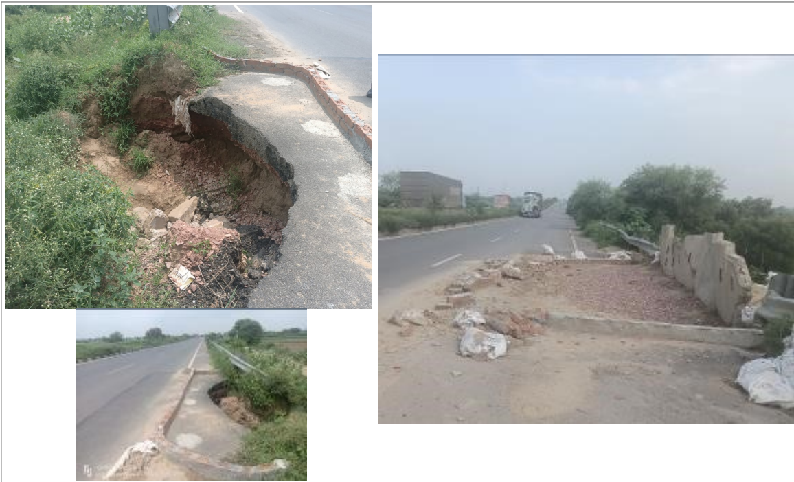
Photo 4: Road subsidence along the National Highway
