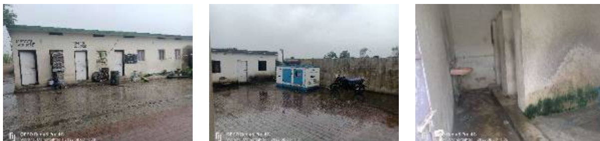
Figure 2-4. Facilities at Darodha Toll Plaza
