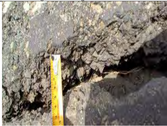
Cracking at Km 44.300 RHS
