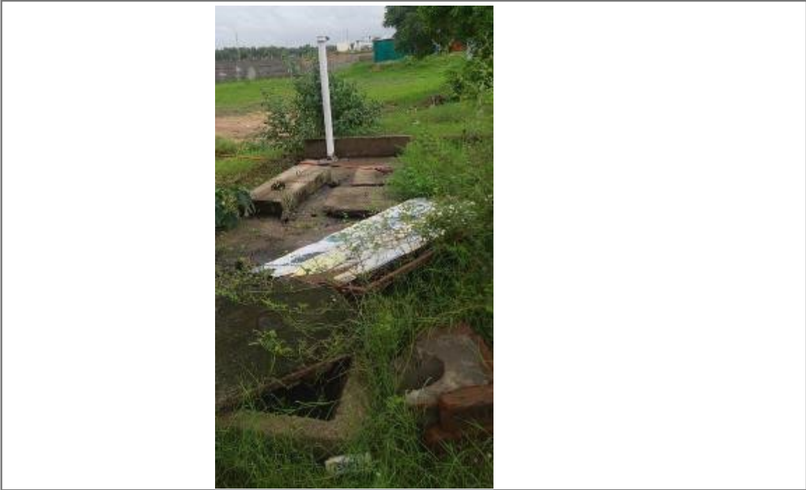
Photo 11: Septic tank in the toll plaza premise
