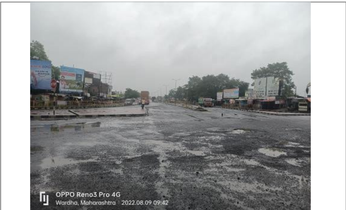
Photo 4: Potholes on the highway
