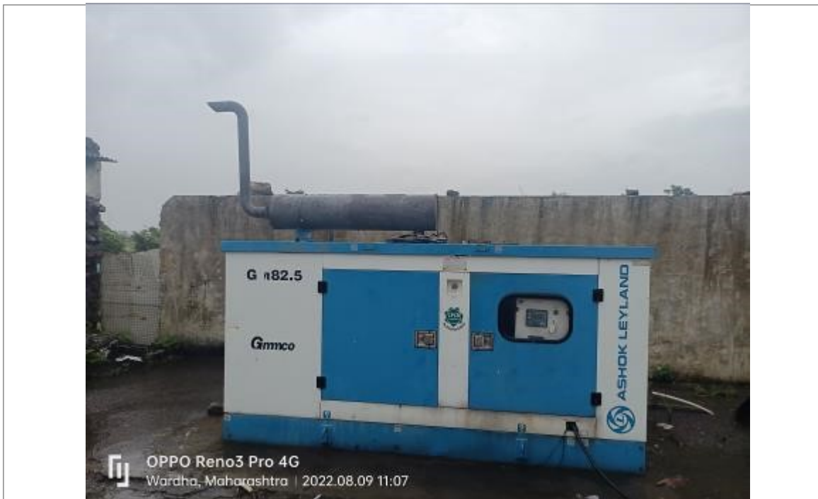
Photo 11: Diesel Generator at the toll plaza
