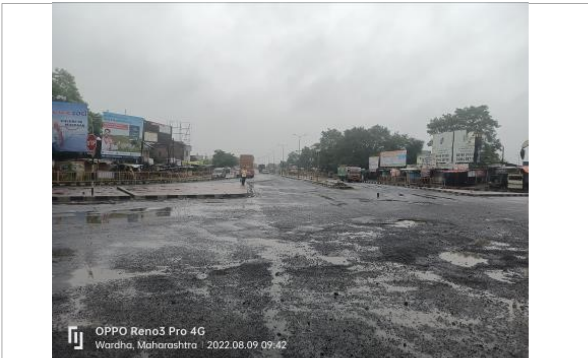
Photo 4: Potholes on the highway
