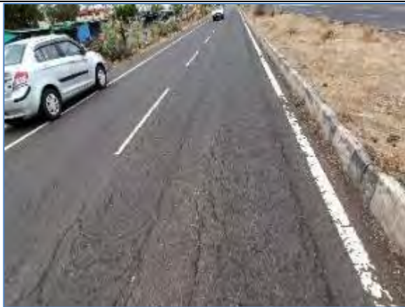
Rutting at Km 113.600 RHS
