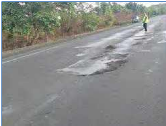
Bleeding & Patching at Km 127.700 RHS
