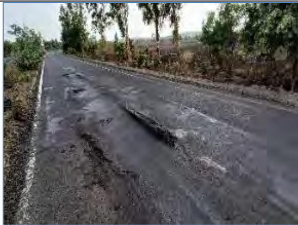
Shoving at km 125.600
