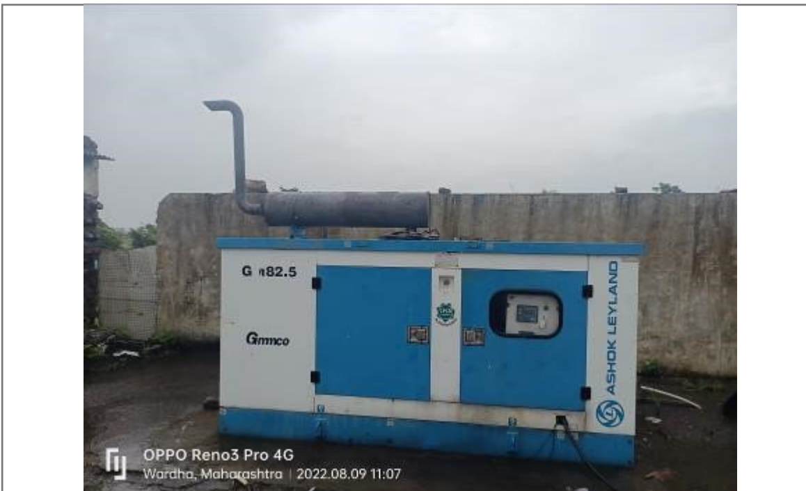
Photo 11: Diesel Generator at the toll plaza
