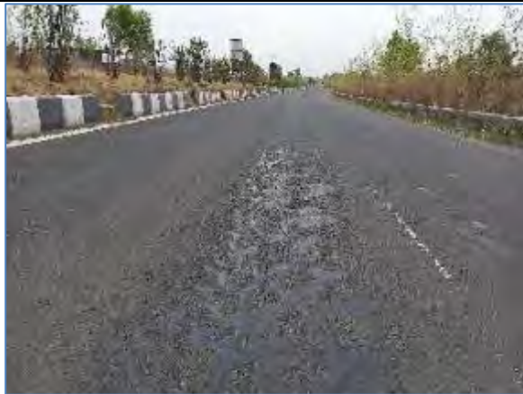
Bleeding at km 92.000-LHS
