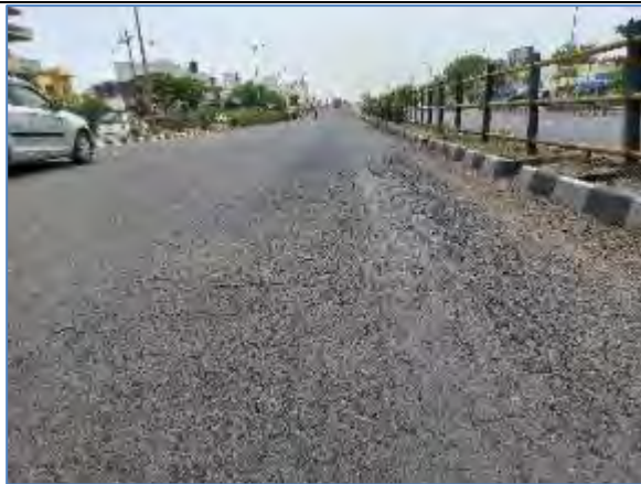
Alligator cracking at km 74.900-RHS
