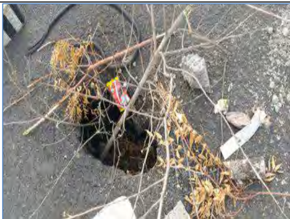
Pothole at Km 43.200 RHS
