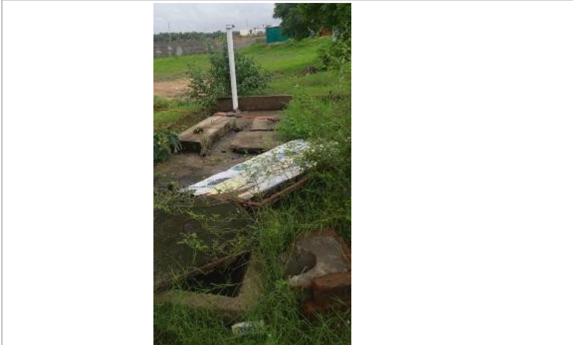
Photo 11: Septic tank in the toll plaza premise
