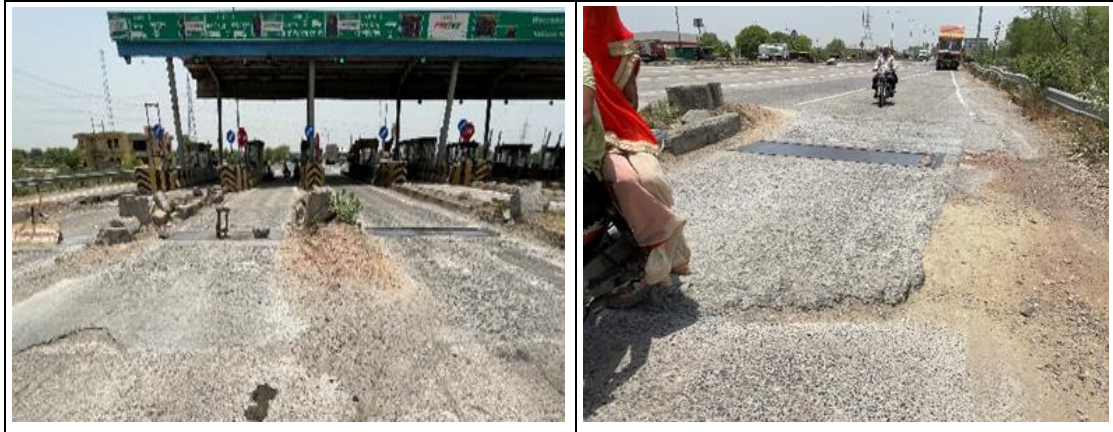
Figure 2.3: Rigid Pavement Condition
