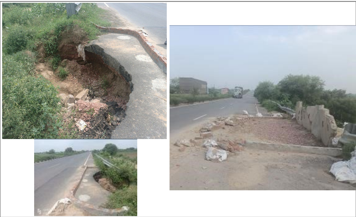
Photo 4: Road subsidence along the National Highway
