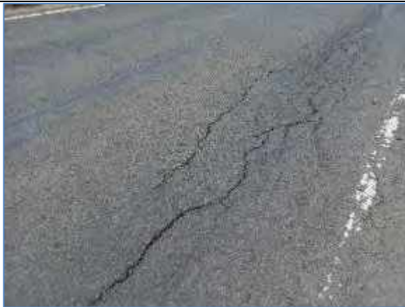
Longitudinal cracking at Km 59.100 RHS
