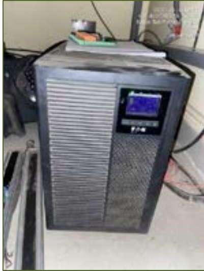
Figure 3-21: UPS at Server Room.
