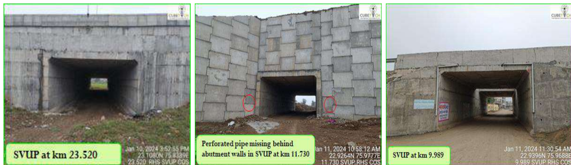
Figure 4-7: Condition of LVUPs
