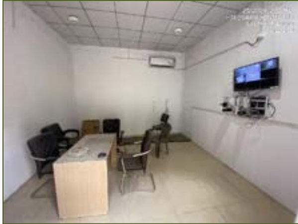
Figure 3-47: Tunnel-2 Control Room.
