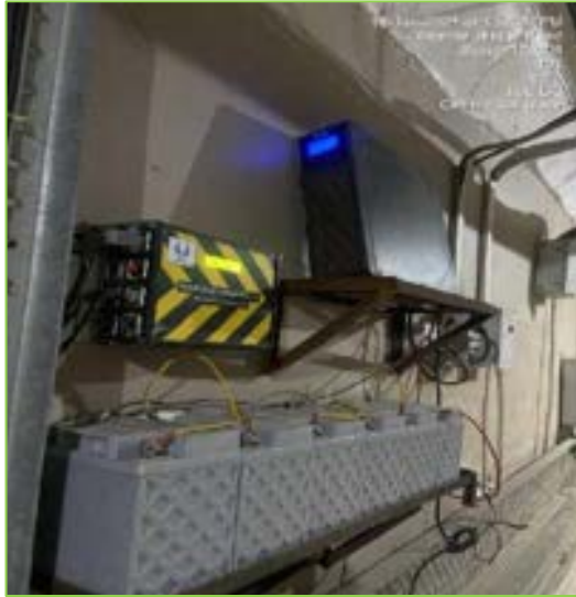
Figure 3-23: Lane UPS in Tunnel.
