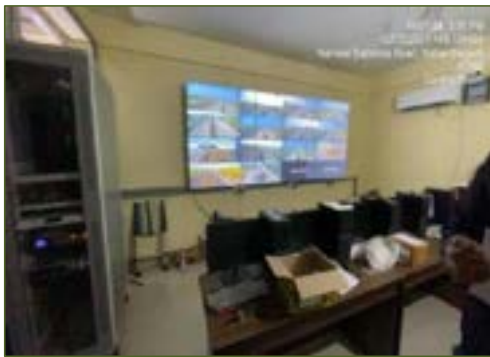
Figure 3-29: Workstations in ATMS control room.
