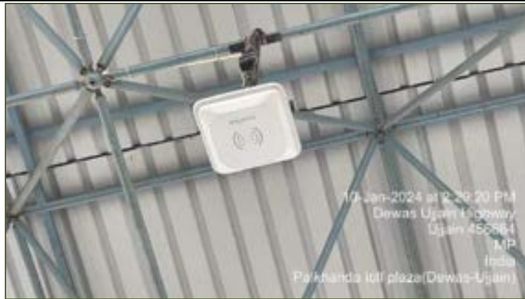
Figure 3-14: RFID ETC Transceiver installed on pole
