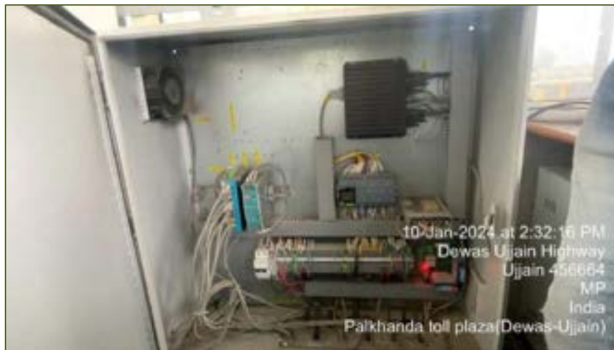
Figure 3-15: Lane Controller at Toll Booth
