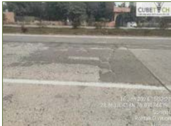
Figure: Tranverse Cracks
