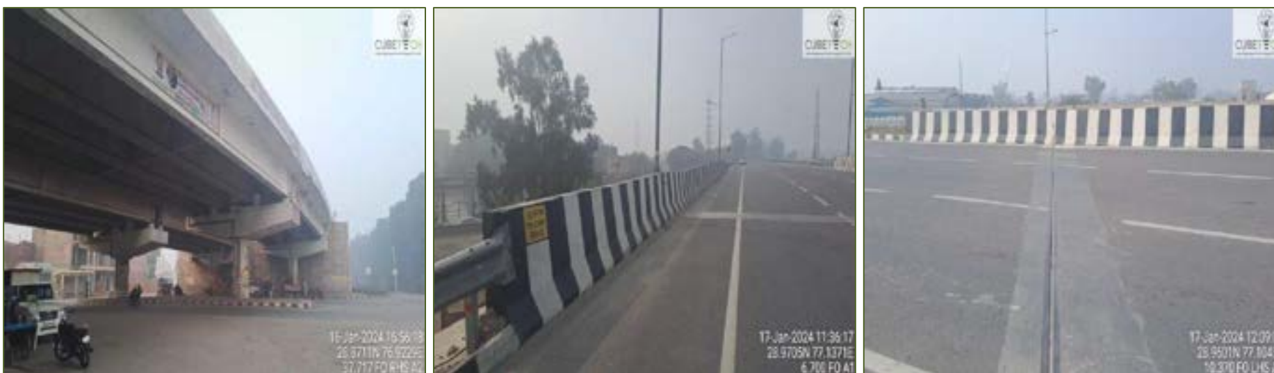
Figure 4-3: Condition of Flyover
