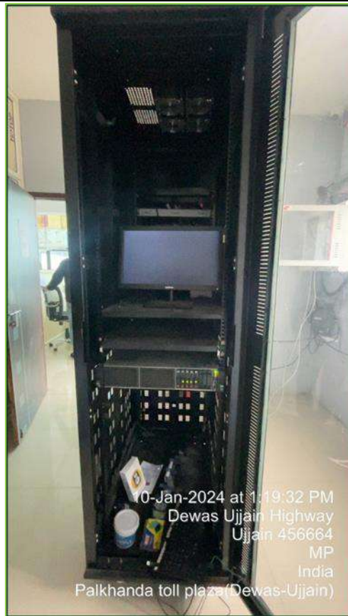
Figure 3-25: Server with rack.
