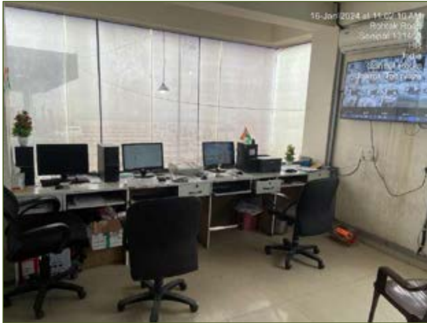
Figure 3-21: Workstations at Control room.
