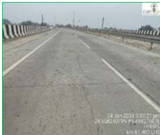
Figure: Longitudinal Cracks
