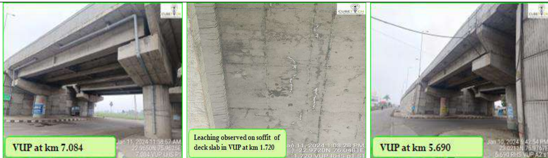
Figure 4-5: Condition of VUPs
