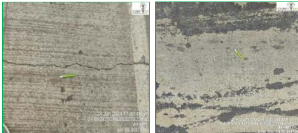
Figure: Transverse Cracks
