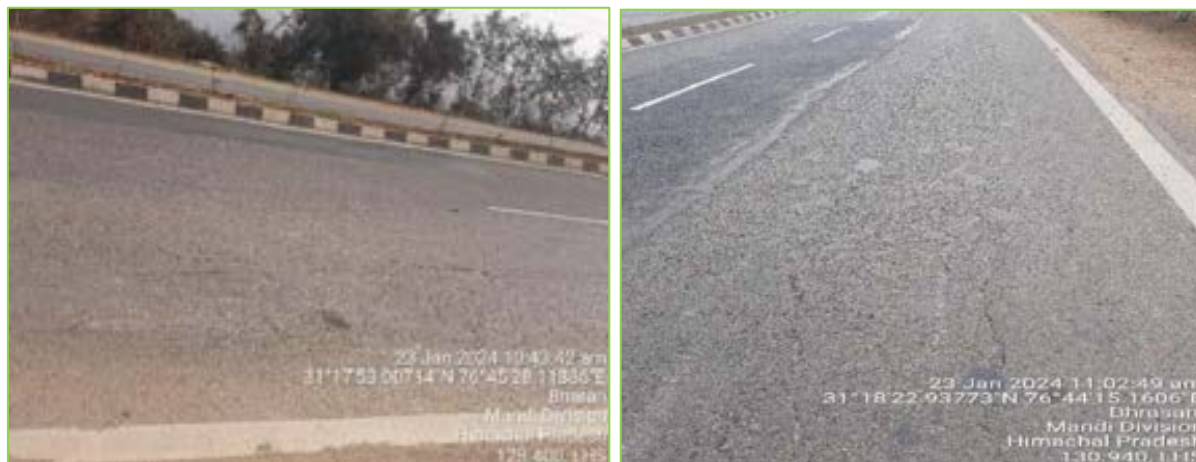
Figure: Alligator Cracks
