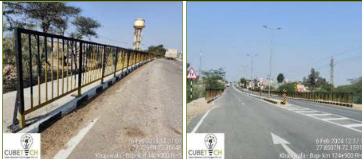
Figure 3-7: Pedestrian guard rail
