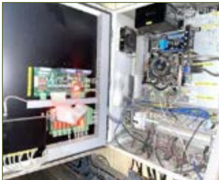
Figure 3-9: Toll Lane Controller inside Tunnel.
