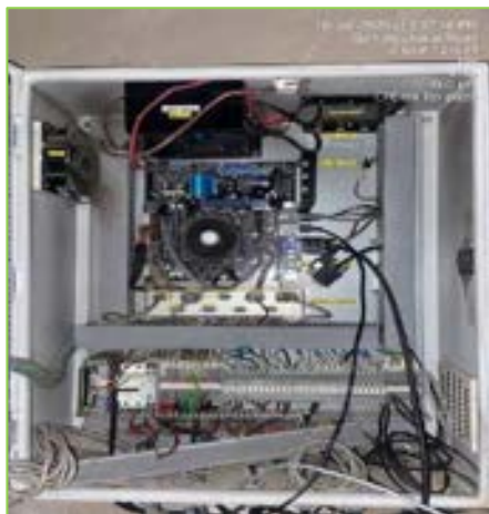
Figure 3-10: Toll Lane Controller at Tunnel
