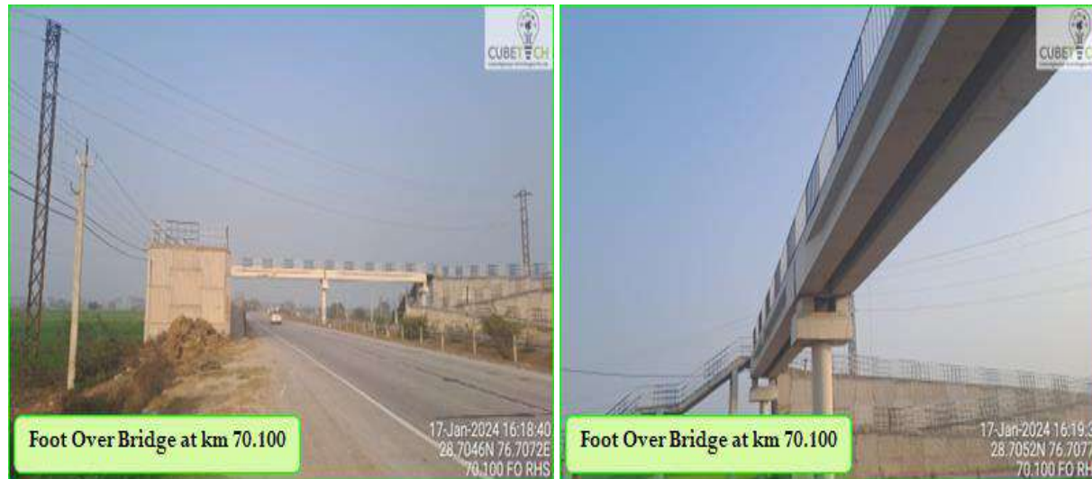
Figure 4-4: Condition of Foot Over Bridge
