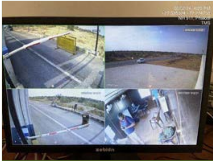
Figure 3-21: Cameras at TP-3
