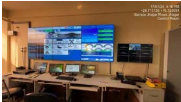
Figure 3-31: ATMS Control Room.
