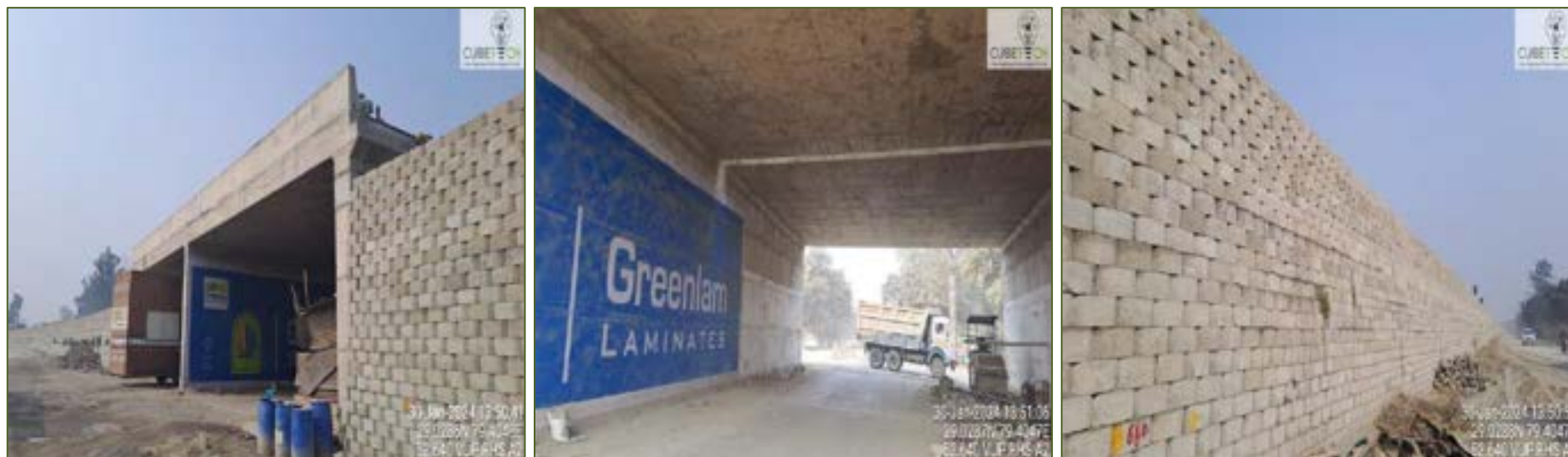
Figure 4-5: Condition of Vehicular Underpass
