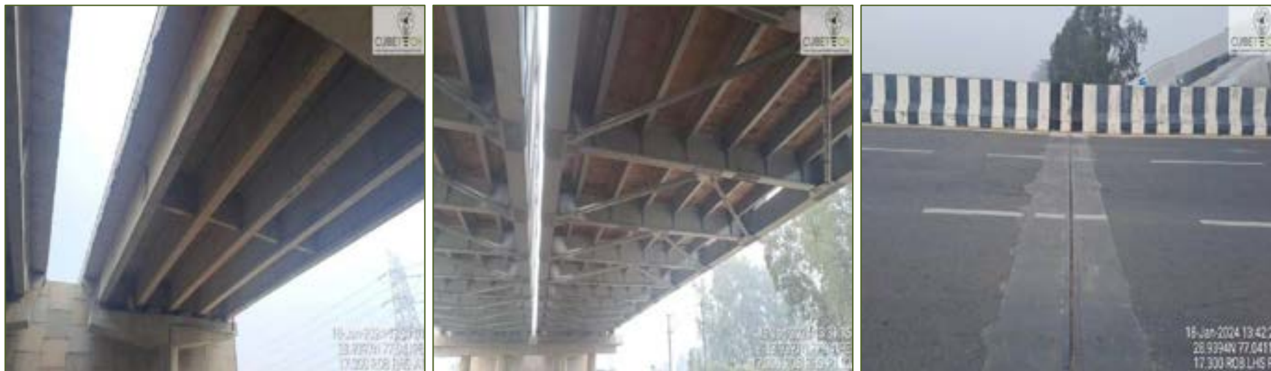
Figure 4-2: Condition of ROB
