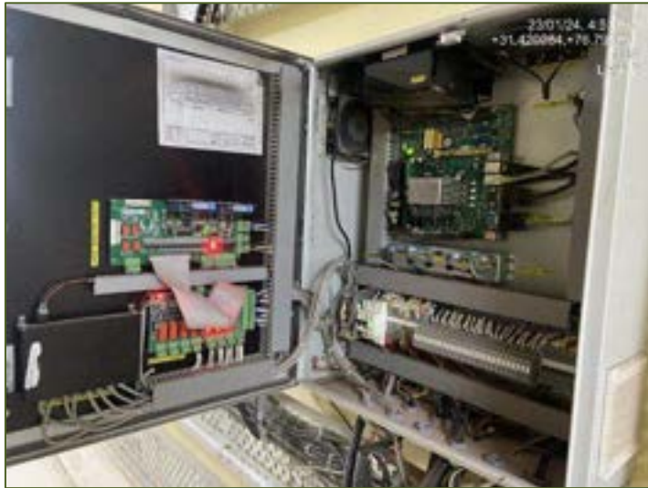
Figure 3-10: Toll Lane Controller inside Tunnel.
