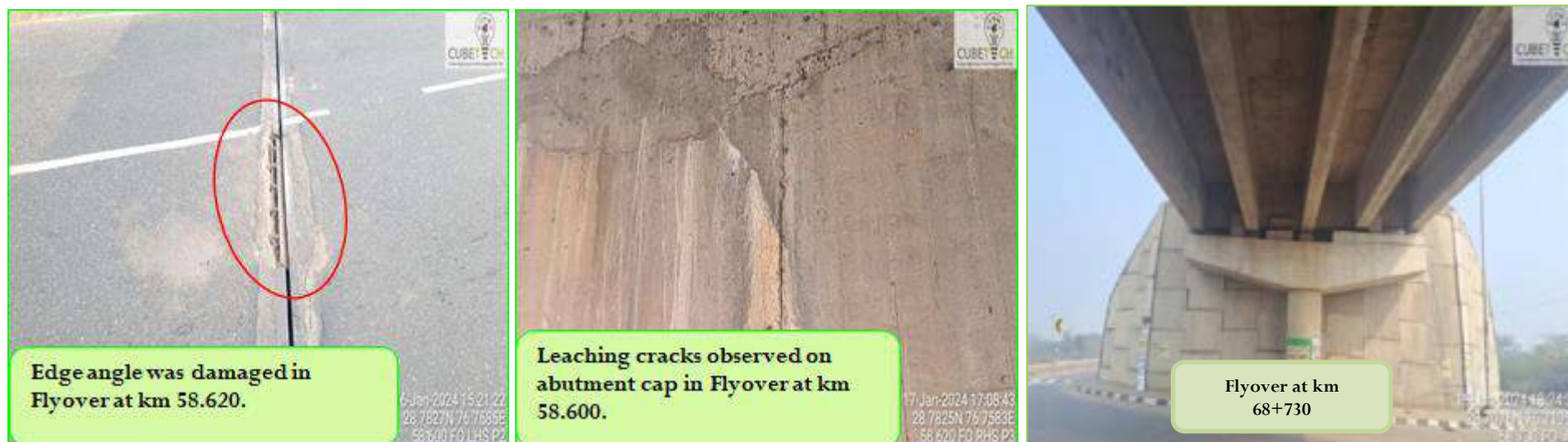
Figure 4-3: Condition of Flyover
