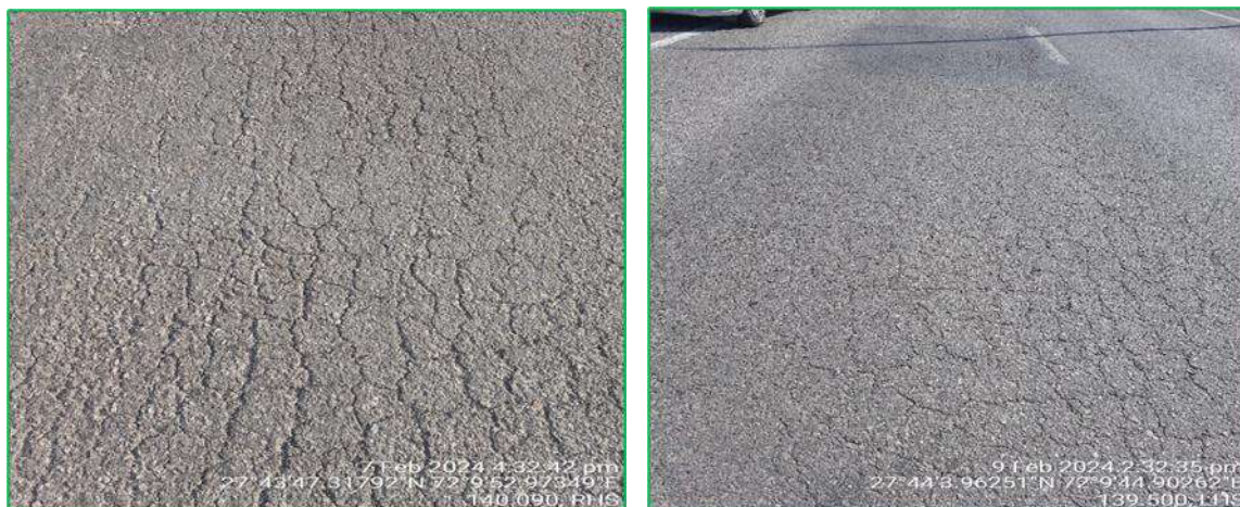
Figure: Alligator Cracks
