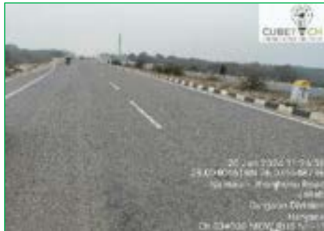
Figure: Longitudinal Cracks
