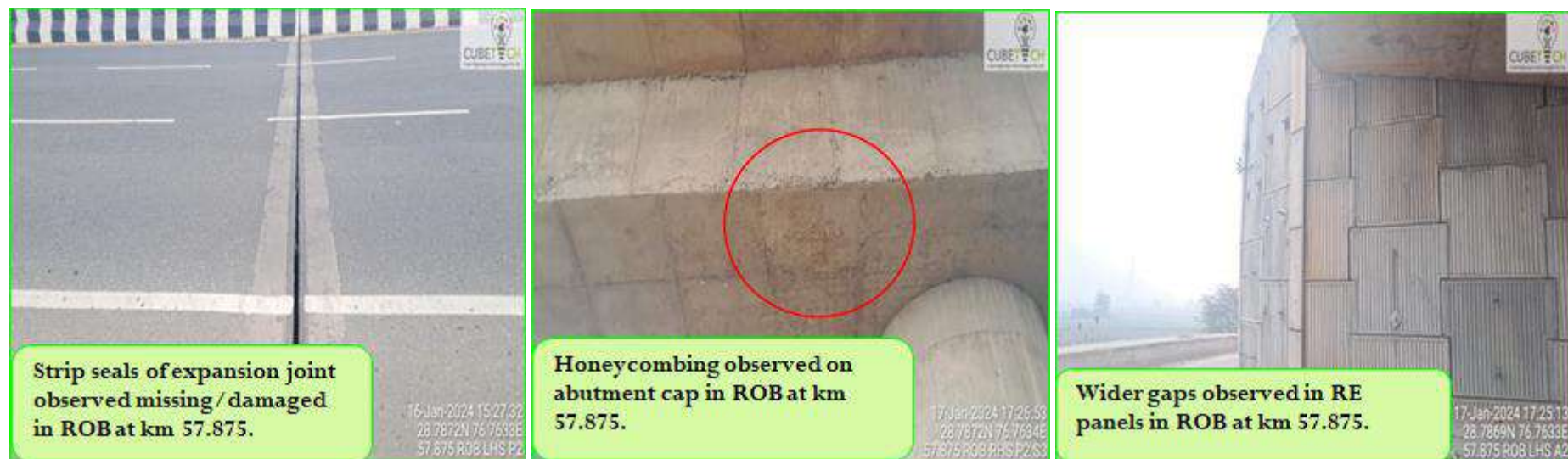
Figure 4-2: Condition of ROB
