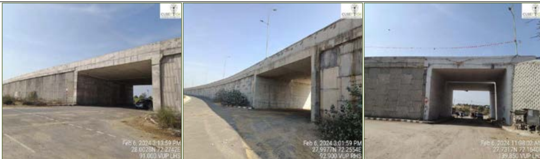
Figure 4-2: Condition of VUPs
