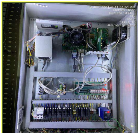
Figure 3-9: Toll Lane Controller at Tunnel
