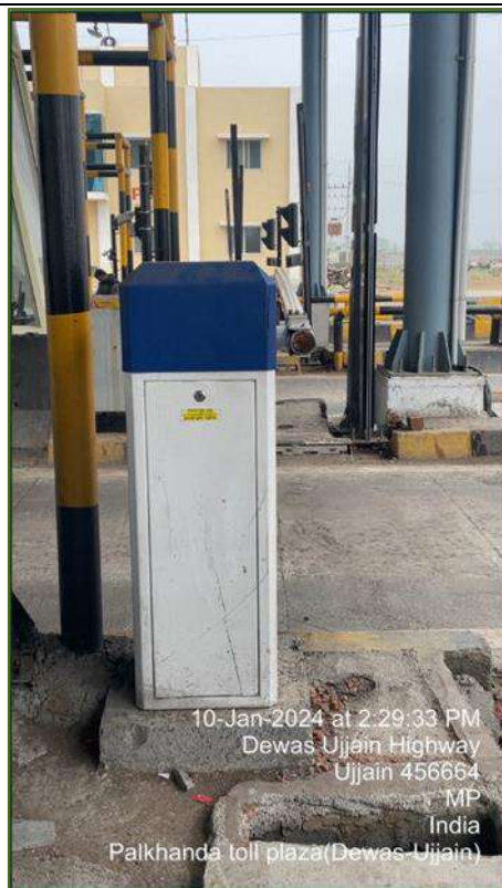
Figure 3-17: Automatic Lane Barrier
