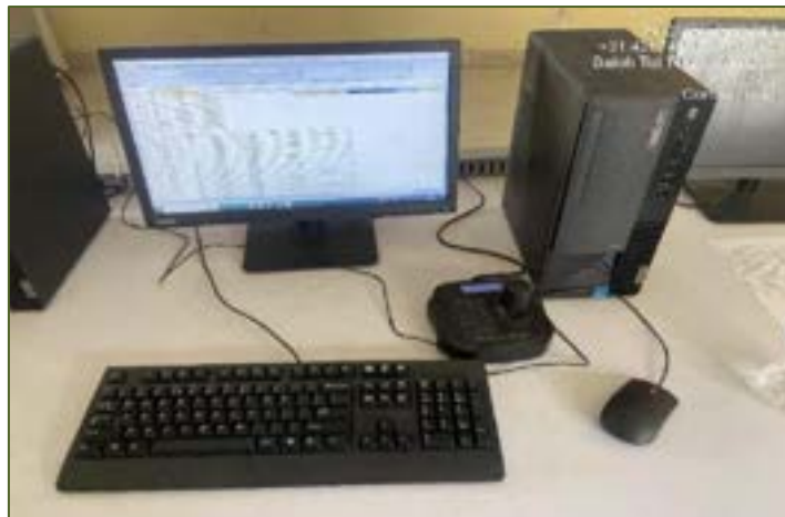
Figure 3-37: Workstations in ATMS control room.
