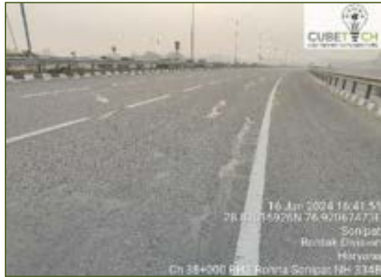
Figure: Longitudinal Cracks
