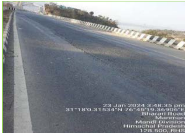
Figure: Longitudinal Cracks
