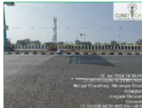
Figure: Transverse Cracks
