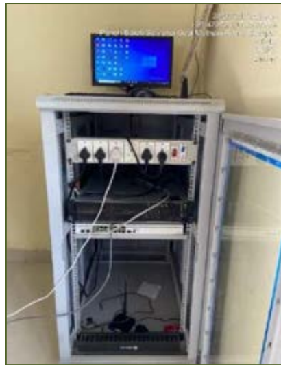
Figure 3-39: ODFS Server with Rack.
