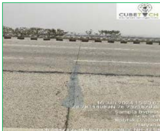
Figure: Spalling of joints
