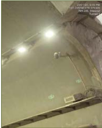
Figure 3-44: Tunnel-1 PTZ Camera.
