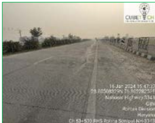
Figure: Longitudinal Cracks
