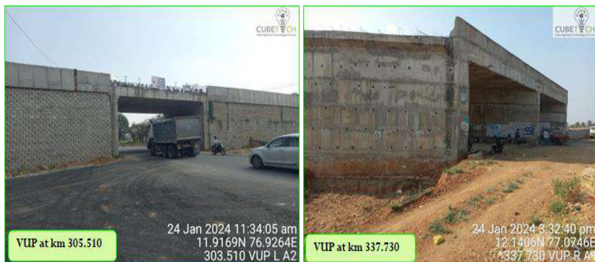
Figure 4-4: Condition of VUPs
