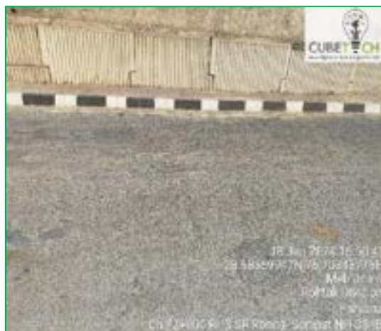
Figure: Alligator Cracks
