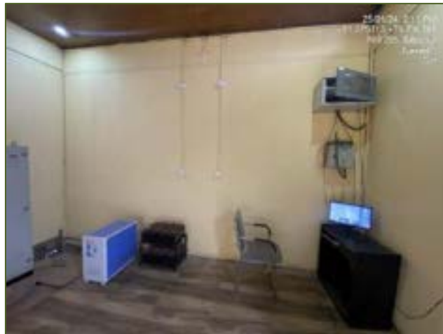
Figure 3-49: Tunnel-3 Control Room.
