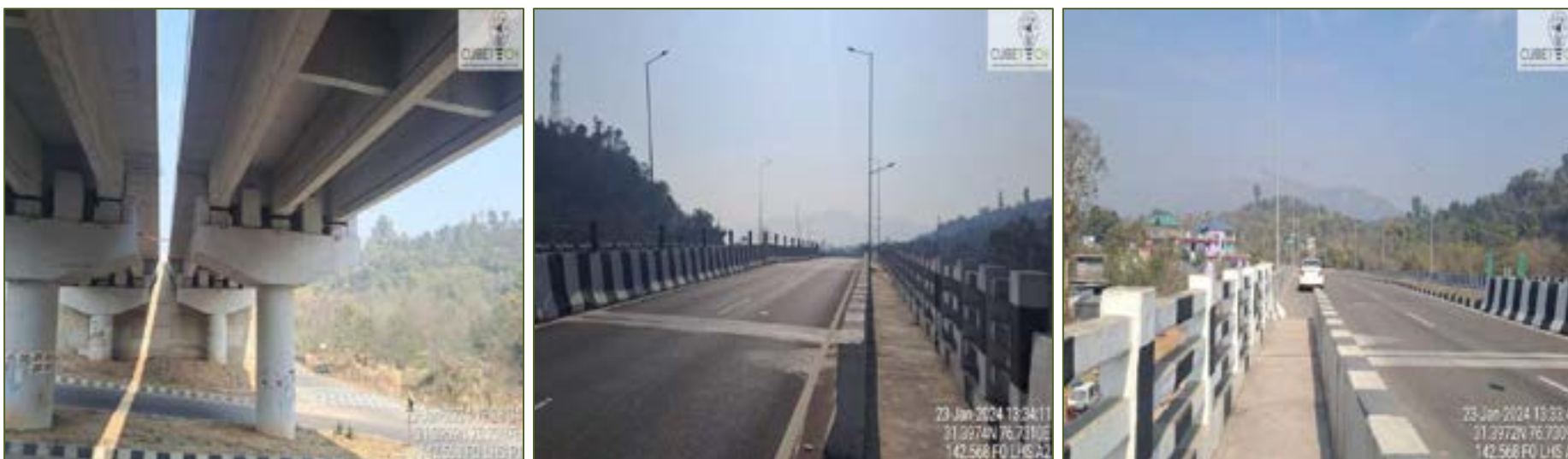
Figure 4-4: Condition of Flyover
