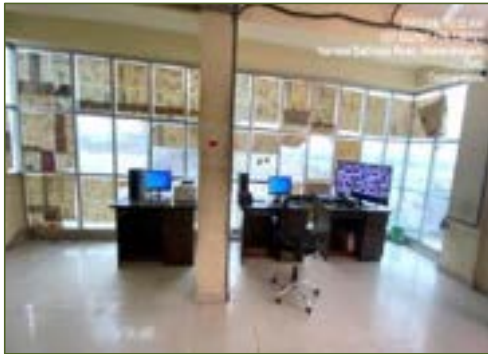
Figure 3-18: Workstations at Control room.
