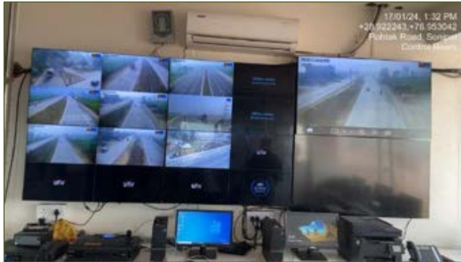
Figure 3-30: ATMS Control Room Equipment.
