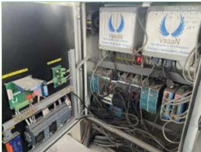
Figure 3-16: Toll Lane Controller inside Booth
