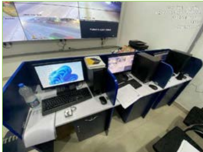
Figure 3-41: Workstations in ATMS control room.
